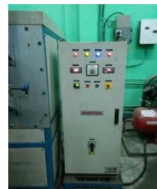
Figure 1(b). Furnace Control Panel
